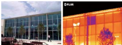
Building diagnostics - Infrared testing is used to detect heating & cooling loss or moisture problems due to insulation deficiencies or construction issues.
