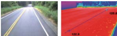
Cooling asphalt mat - With only a 3 Fahrenheit degree differential, the longitudinal section shown in the thermograph indicates that this cooling asphalt mat exhibits exceptional thermal uniformity. The mean density of this asphalt mat is 2,205 kilograms per cubic meter, with a maximum of 2,247 kg/m 3 and a minimum of 2,179 kg/m 3 . The visual photo of the road taken a year later shows no evidence of wear or degradation.
